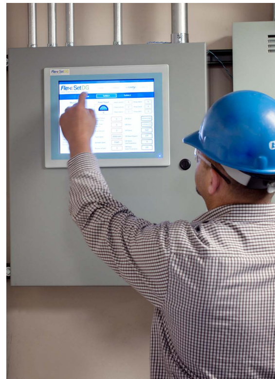
FlexSetDG controls for distributed generation systems allow 24/7 remote equipment monitoring.
